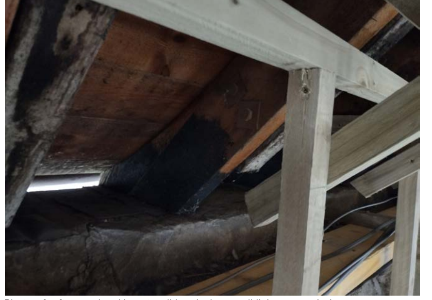
Photo of rafters and sarking at wall head where wall linings are missing
